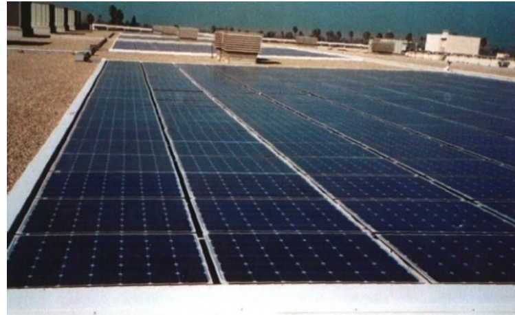
8MW Solar Photovoltaic
