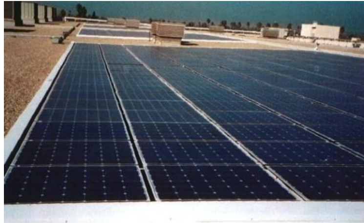
8MW Solar Photovoltaic
