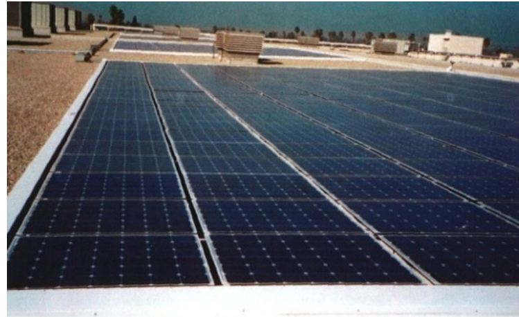
8MW Solar Photovoltaic
